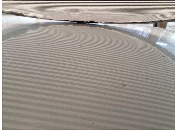
Damage 4: Roof: Roof - Dent(s) - Smooth repair work
