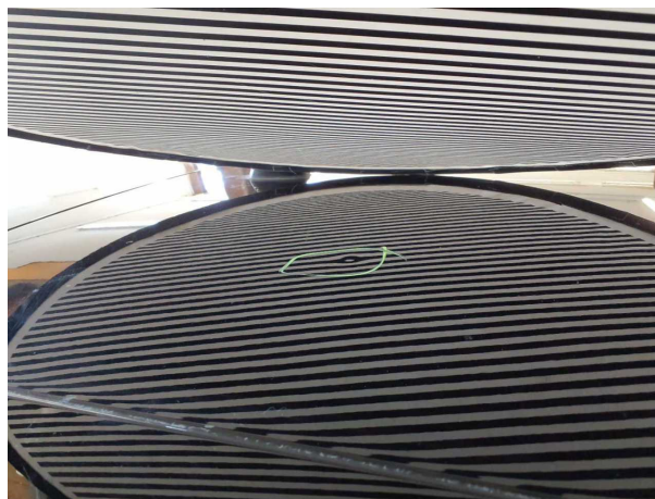
Damage #4: Roof: Roof - dent(s) - Smooth repair work
