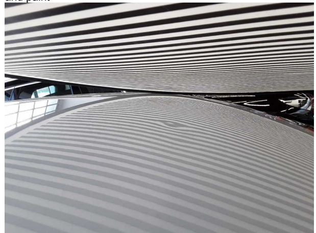
Damage #11: Roof: Roof - dent(s) - Repair and paint
