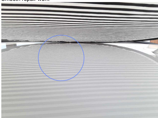
Damage #3: Roof: Roof - dent(s) - Smooth repair work
